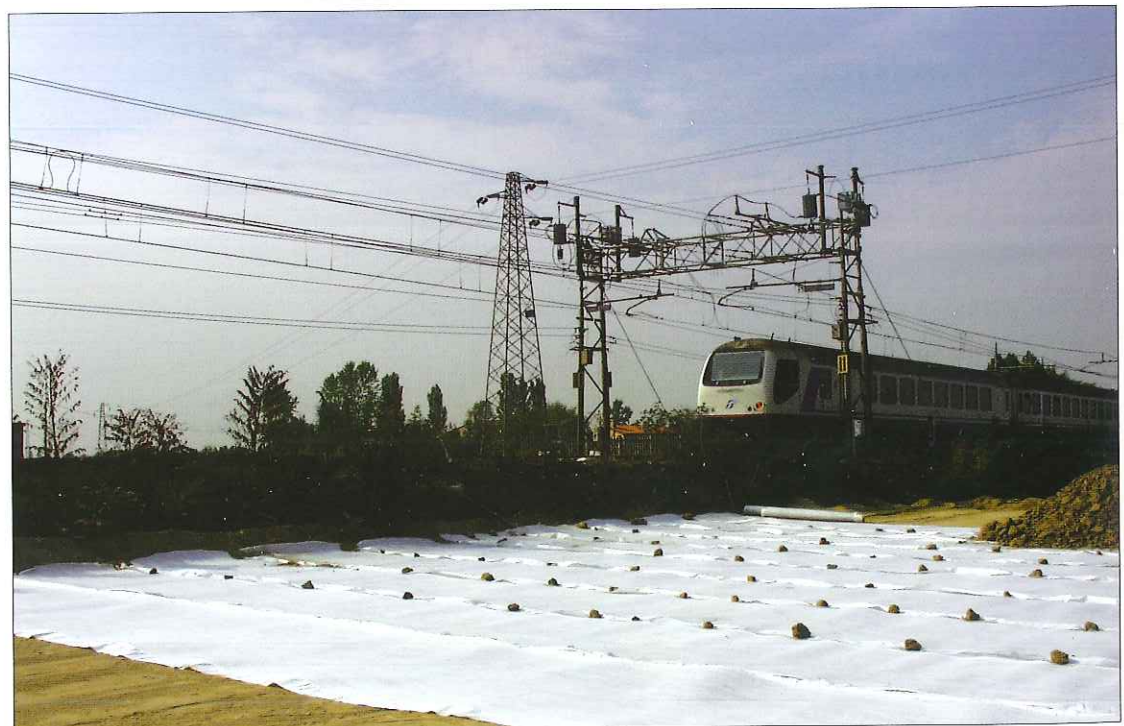
Padova-Mestre, Italy. Capillary break layer under the new high speed train line Milan-Venice in the Venice-Mestre area.
